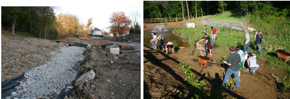
Figure 3. Construction of the stormwater diversion channel in fall 2009; wetland planting by students in spring 2010
