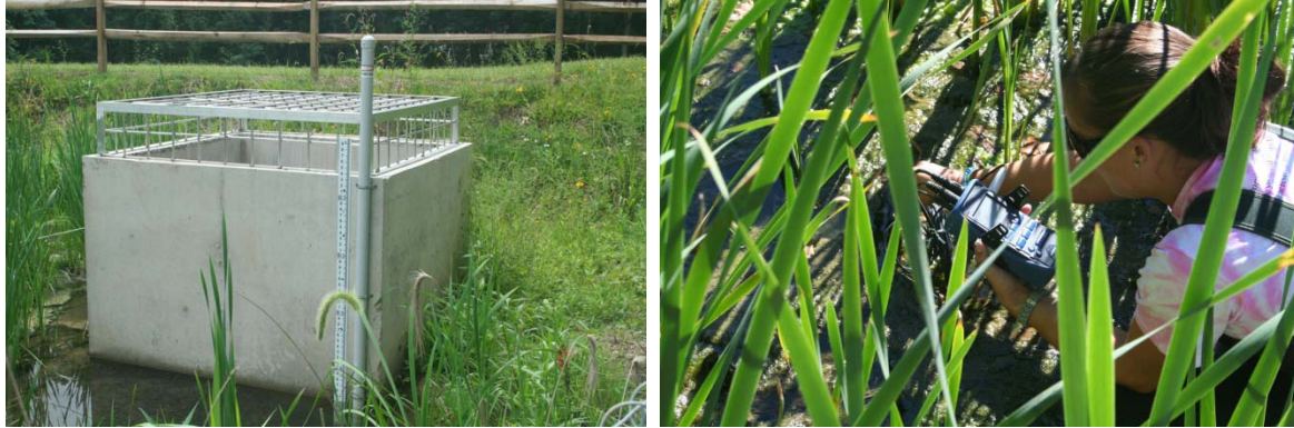
Figure 4. Installation of continuous flow monitoring system in summer, and water quality monitoring in fall 2010
